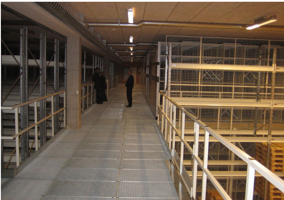
Figure 11. The interior of the Ribe storage has a 6 m ceiling height and mezzanine with racks and compactors. The ducts below the ceiling is for inlet of dry air for humidity control in summer. Photo: Poul Klens Larsen.
